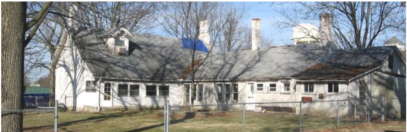
2006 before work started. Bad roof, structural problems, but huge possibilities!
